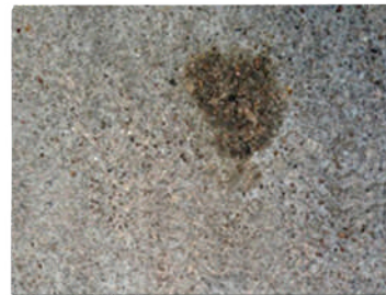
Oil on concrete before treatment
